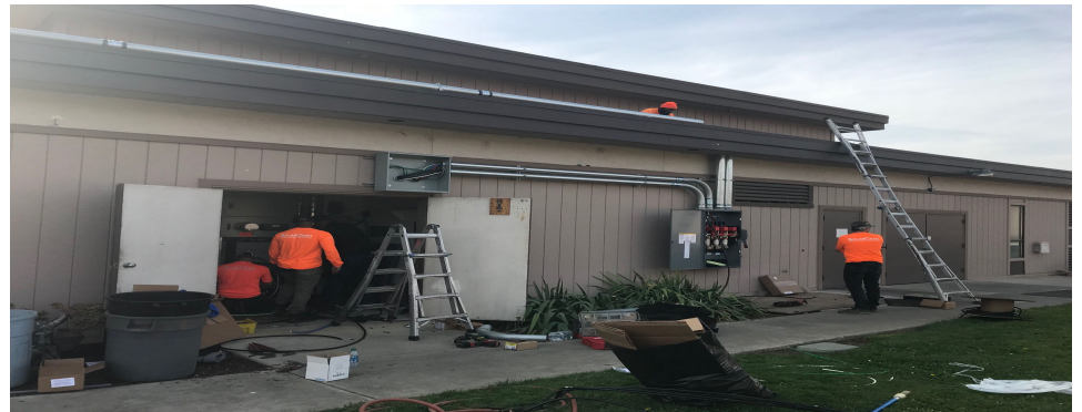
Solar Craft & PG&E working hard to get our solar done by the end of this month.
